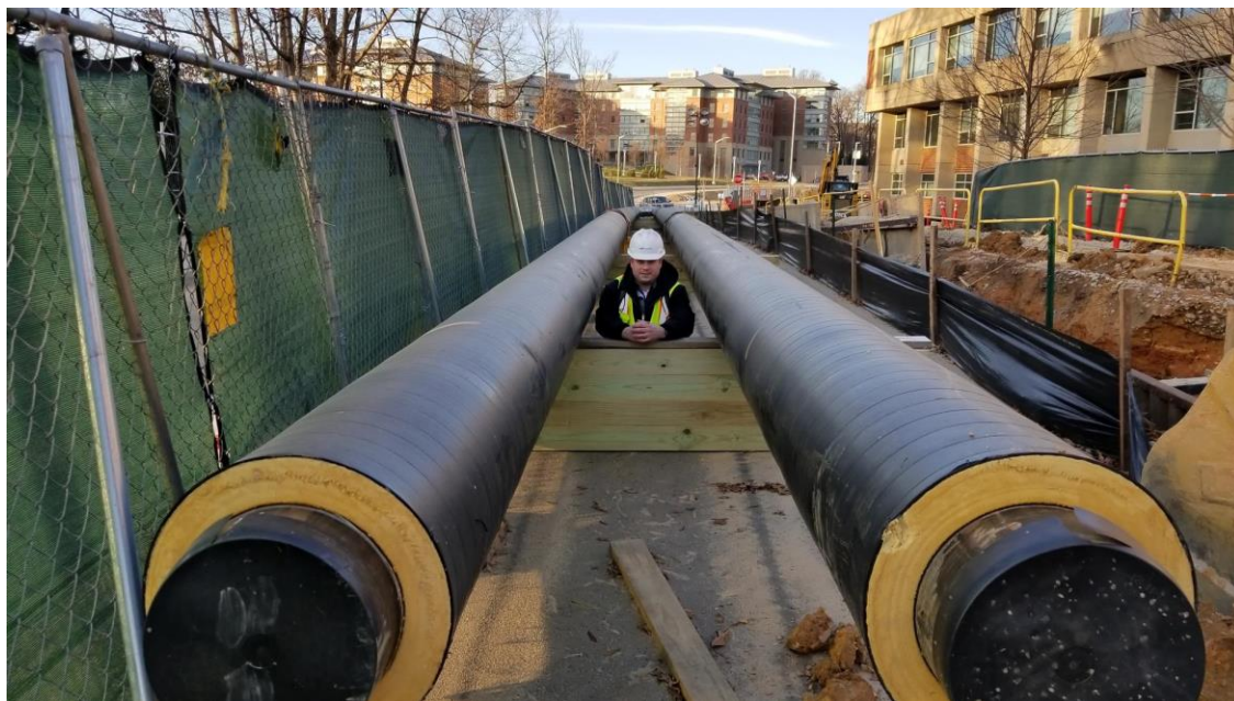
Figure 3 – Insulated and Jacketed Chilled Water Supply and Return Piping
